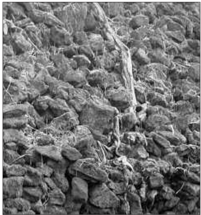
Figure 5. The foundation structure and original wall of first platform on the South side (Photo Paul Wallin)
